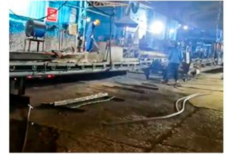
T/Y Post Wire Workshop
